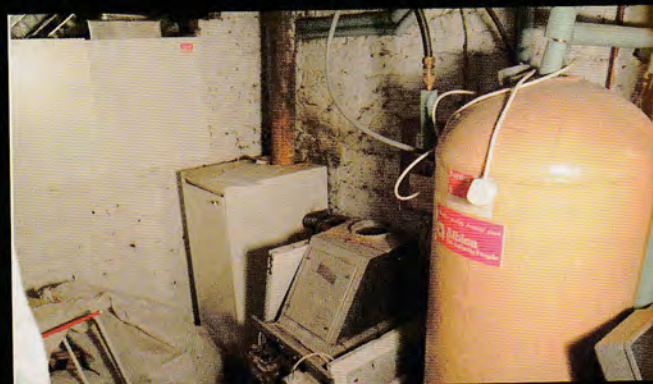
The culprit: the boiler unit located in Miller’s cellar keeps the temperature at a steady, overly warm, 20°C
